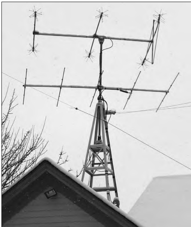
Figure 26.14 — A roof mounted tower will give your antennas a chance to get up in the air with a minimal impact and cost. (Photo by Redd Swindells, AI2N)
