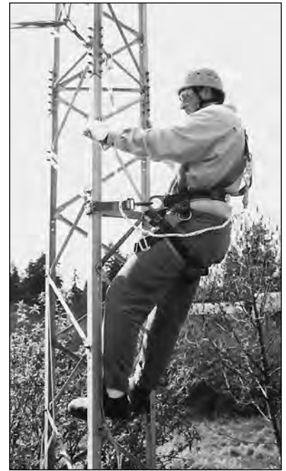
Figure 26.4 — A climber on a tower. Note the fall arrest lanyard attached to the tower above him.
