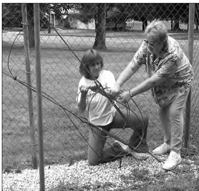
Figure 26.42 — A length of guy cable is used to assure that the turnbuckles do not loosen after they are tightened. This procedure is an absolute requirement in guyed tower systems, as shown by Jodi Morin, KA1JPA (left) and Helen Dalton, KB1HLF.
