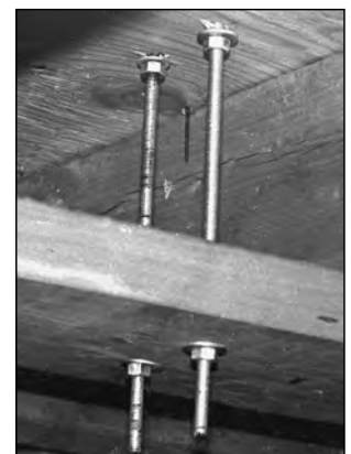
Figure 26.15 — The strengthened anchoring for the roof-mounted tower. Bolts run through the roof and through the anchor plate (2 × 6) between joists. (Photo by Jane Wolfert)
