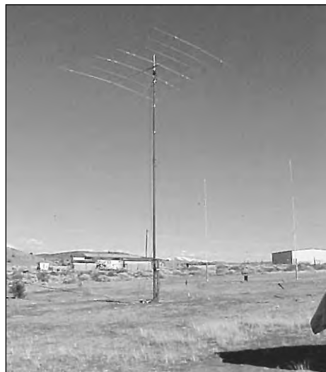
Figure 26.9 — Installation of surplus AB-577 tower with tribander at 45 feet at K7NV. (Photo by Kurt Andress, K7NV)
